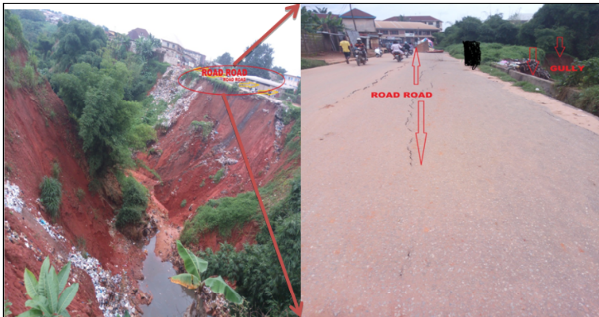
Fig.4: The Gully Encroaching a Major Road
