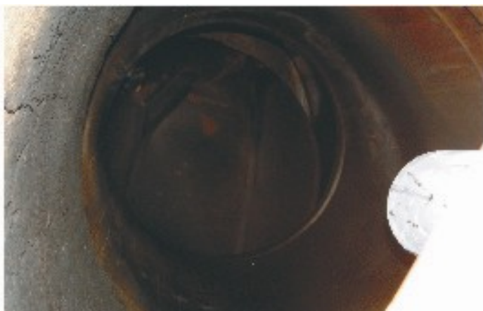
Figure 4: Corrosion Effects in Burner Internal
