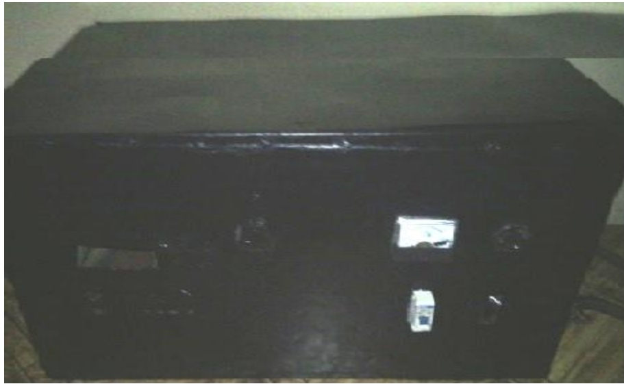
Figure 3: AC Power Generator System
